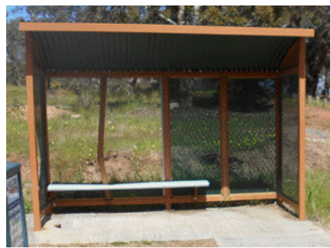
Steel bus shelter (Miricale) with vandalised panels
