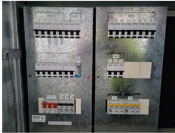
Figure 9-6: Distribution Board in the Rollerama
