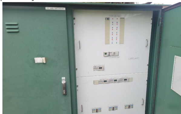
Figure 9-4: Main switch board
