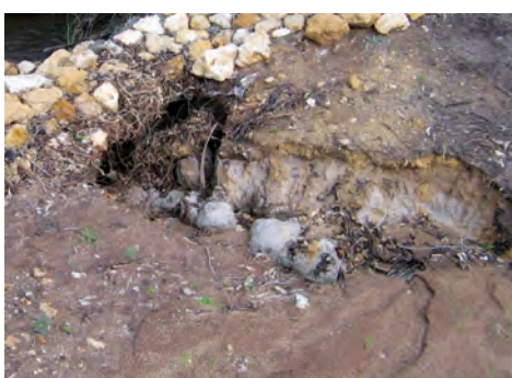
The new erosion management rock banks at Yule Brook have failed and need reviewing and repair.
