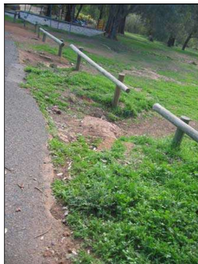
Figure 22: Poor access at edge of carpark
